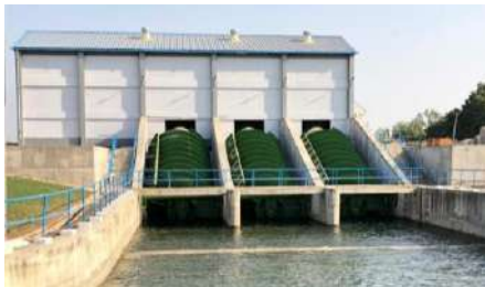
Hydropower Screw Generator
