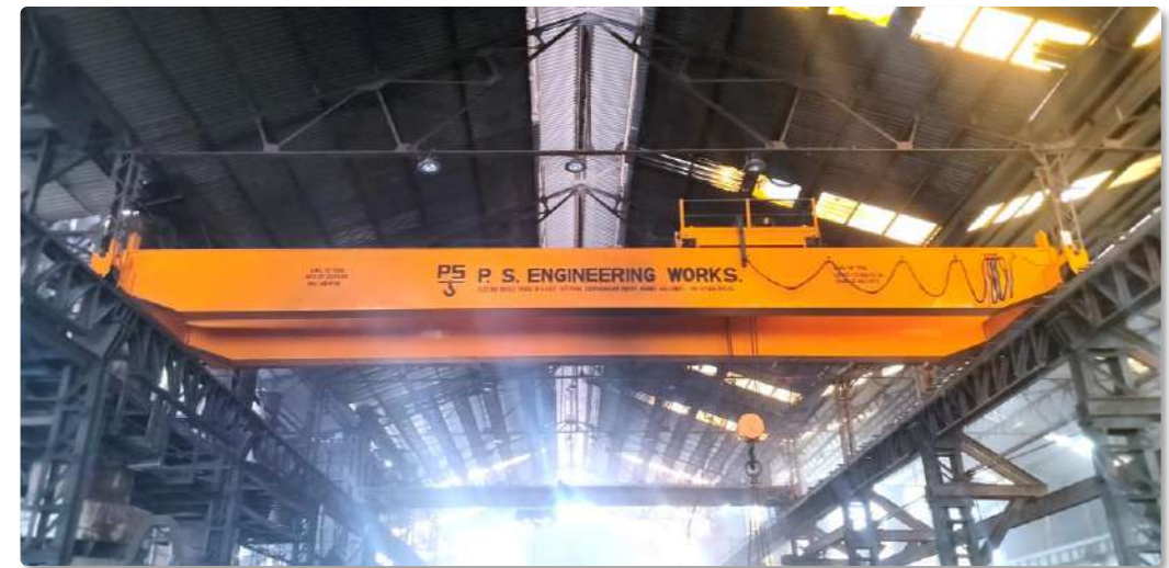
15 T capacity crane installed at Unit 1
