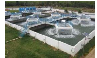
Slow speed fixed aerator
