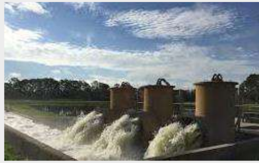
Storm water pumping stations
