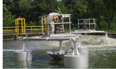
Slow speed floating aerator
