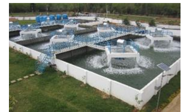
Slow speed fixed aerator
