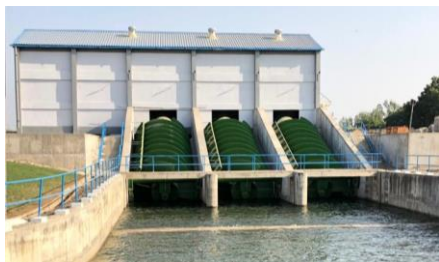
Hydropower Screw Generator
