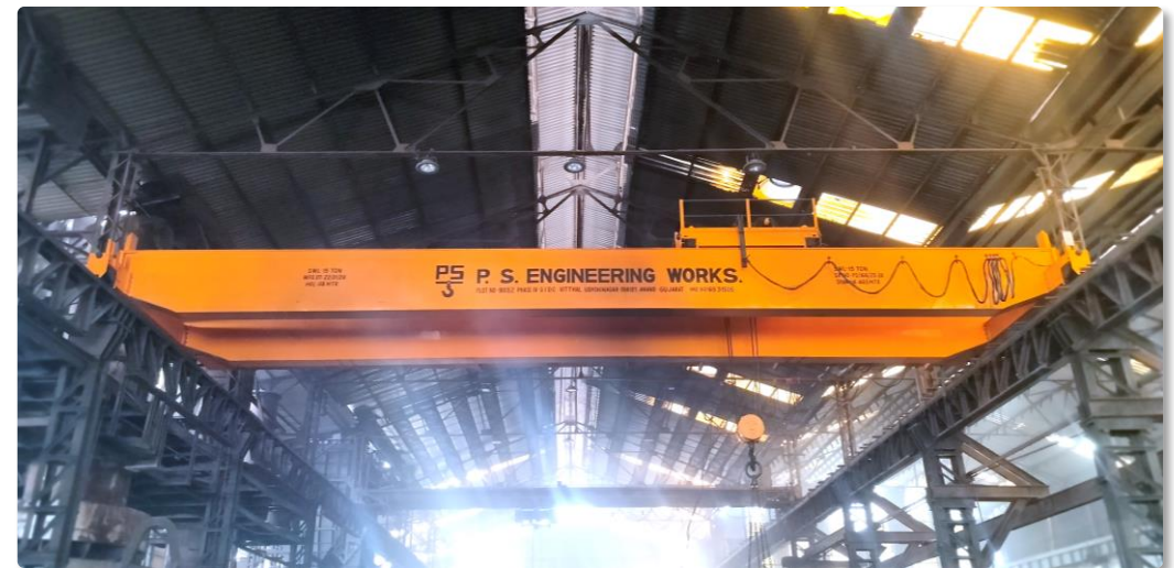
15 T capacity crane installed at Unit 1
