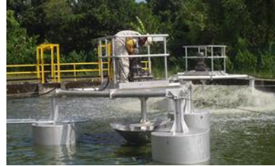
Slow speed floating aerator
