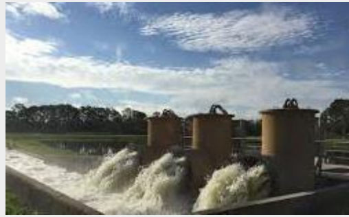
Storm water pumping stations
