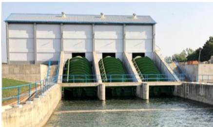
Hydropower Screw Generator
