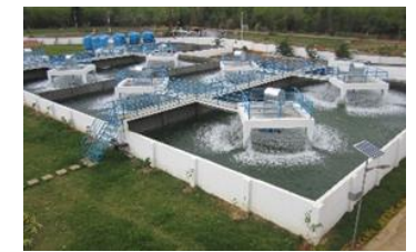
Slow speed fixed aerator
