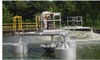
Slow speed floating aerator
