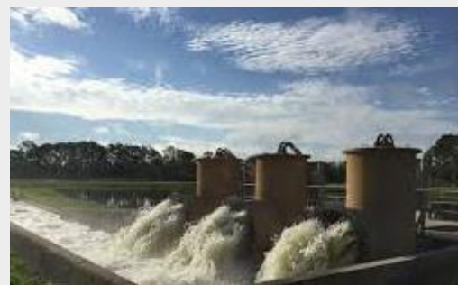
Storm water pumping stations
