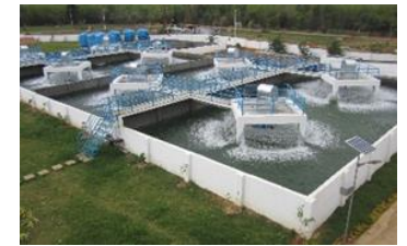
Slow speed fixed aerator
