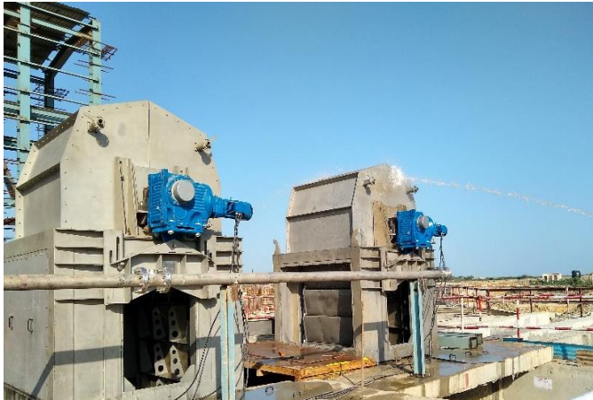
Screens at RSPL Sea Water Intake, Dwarka, Gujarat, India.
