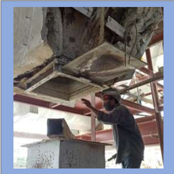
Damaged Isolation Valve at Customer's End.
