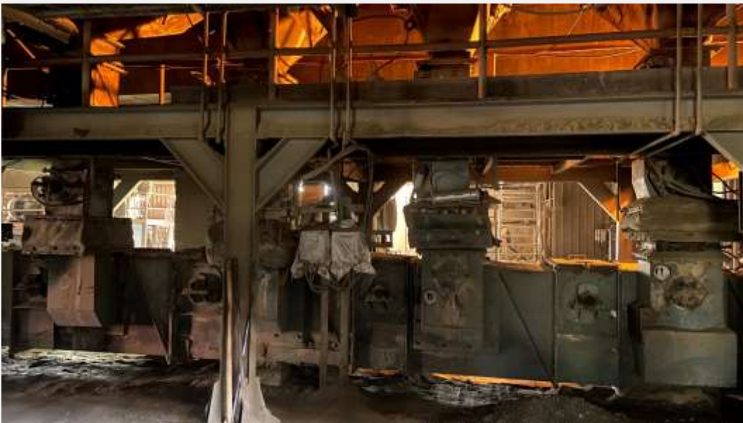
Installation of our Double Flap Valve DFG 300 along side existing fabricated double flap gate.
