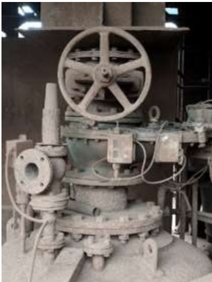
KU-PAM DN250 Installed at M/s Bhilai Steel Plant
